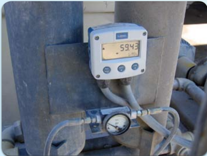
Lube Oil Flow Monitoring with Fluidwell
