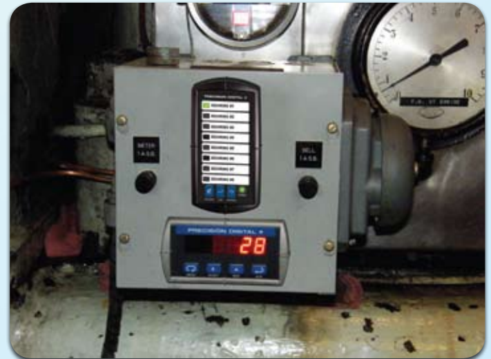
Bearing Temperature Monitoring on a Ferry
